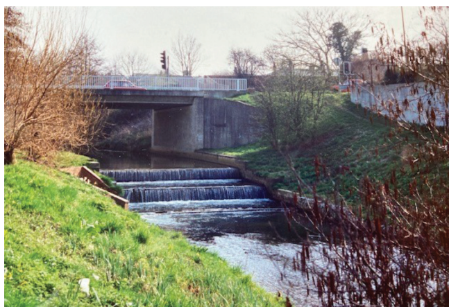
Fig. 13: St Georges Approach Bridge 11 th April 1996. The sampling site is above the weir and beneath the bridge. The scrub on the east bank has now matured.
